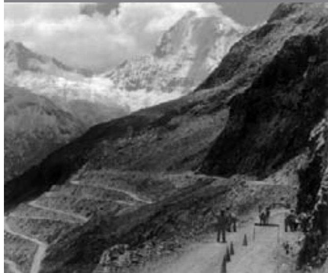
One of 400 microenterprises created under a World Bank–Inter-American Development Bank rural road project, with the participation of men and women from poor rural communities, performs routine maintenance on a rural road in the Peruvian Sierra.
