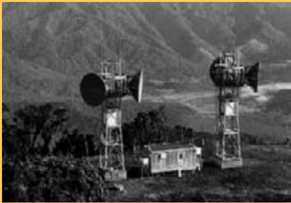
A microwave relay station atop Mt. Chingal (elevation 9,000 feet) near Lae, Papua New Guinea, part of a 1968 telecommunications project.
