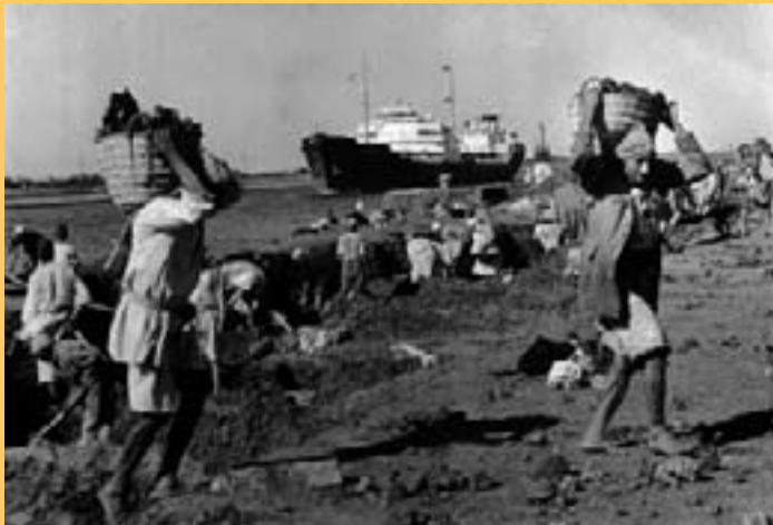
Workers remove soil from the banks of the Suez Canal as part of the 1974 Suez Canal Rehabilitation Project to widen and deepen the canal.
