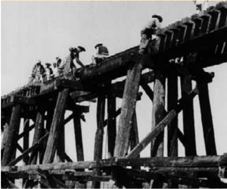
c. 1955. Workmen repair bridges, relay track, install new ties, and rebuild along the Pacific railroad in Mexico. The Bank also financed the purchase of railway stock.
